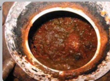
Iron oxide corrosion that builds up on the interior surfaces of glass-lined reactor jackets can be removed with GLRx as part of the ReStor program.
