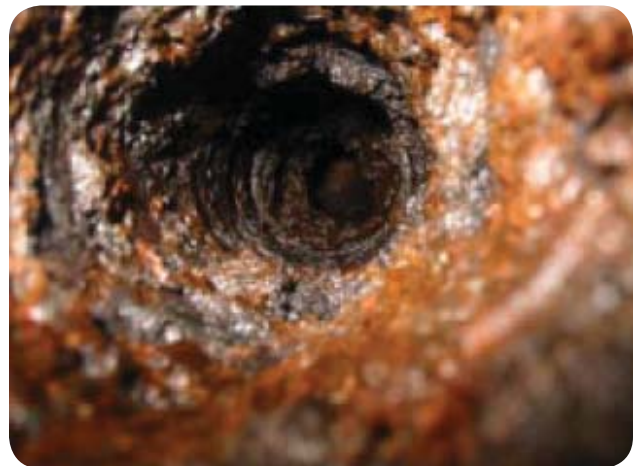
Before cleaning, iron oxide deposition decreases efficiency.
