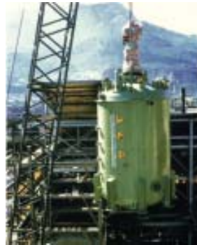
Right: An SA-8000 in final assembly at the De Dietrich facility in Corpus Christi, Texas
